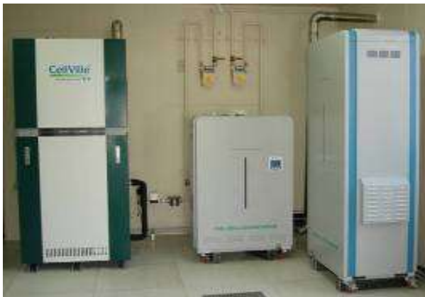
❖ Daegu City Gas (3units, '07.3.12)
