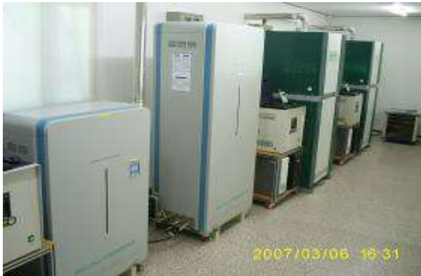
❖ Chungnam City Gas (3units, '07.2.3)
