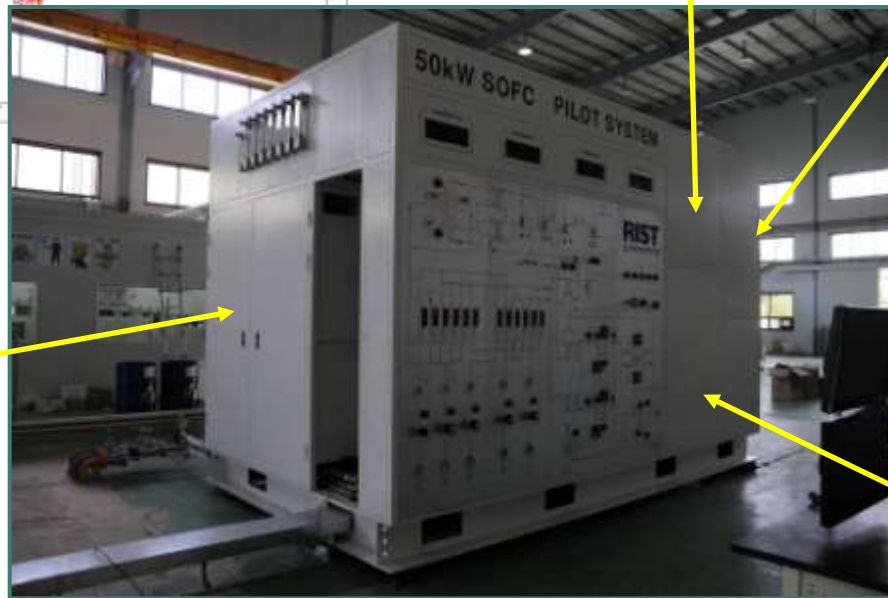
Pilot System (25~50kW)
