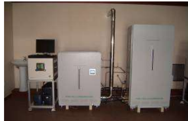
❖ Haeyang City Gas (3 units, '07.4.6)
